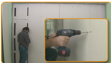
Fix the second gypsum board by using a suitable adhesive. Offset the first board with the second
