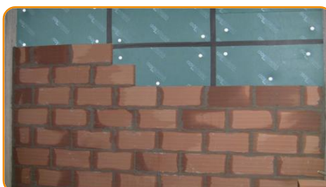
Build up the second wall by caring to joint the blocks with mortar on both vertical and horizontal joints.
