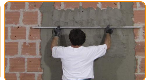
Apply in the first wall a layer of row mortar of about 1 cm thickness
