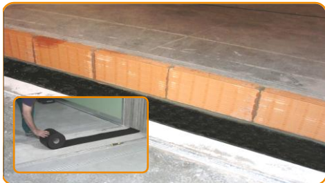
Lay the under wall strip in the dry floor before to build the wall.
