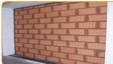
Build up the wall by caring to joint the blocks with mortar on both vertical and horizontal joints.
